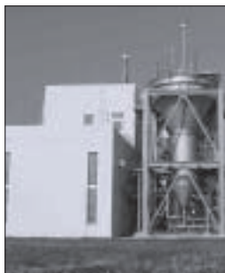
Commerically operational full-scale struvite recovery installation at Shimane Prefecture sewage works. Photo : Unitika Ltd, Japan.
