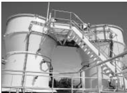
The full-scale calcium phosphate recovery installation at Geestmerambacht sewage works, The Netherlands, was visited by Conference participants. Photo : DHV, Amersfoort,
